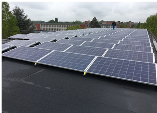
IPES Hesbaye – Installation photovoltaïque
